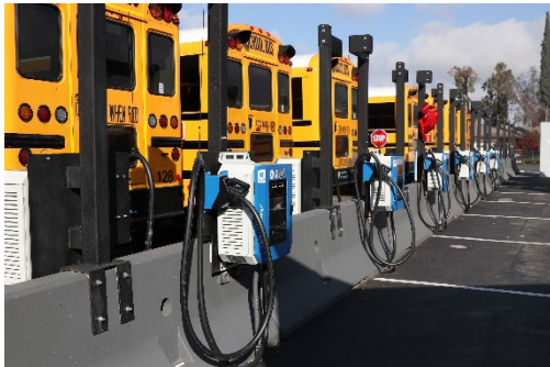
Moreno Valley Unified School District features electric school buses and charging stations
