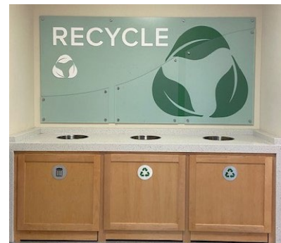
East Providence High School features built-in recycling station.
