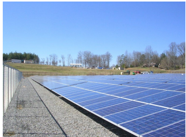
Martins Creek Elementary School – Solar Array Photo credit: ESA Renewables, LLC
