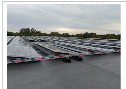
Cambridge Elementary School features solar panels on the roofs of the pool and library.
