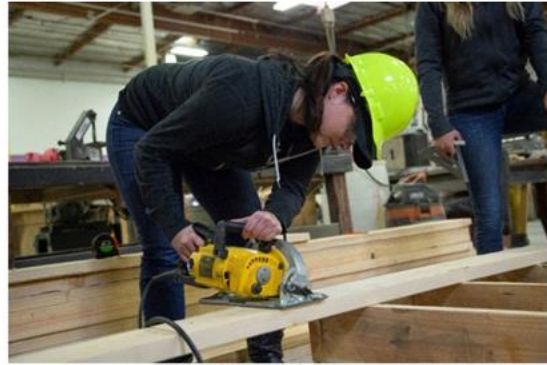
Truckee Meadows Community College students construct a life-size sustainable homeless shelter prototype.
